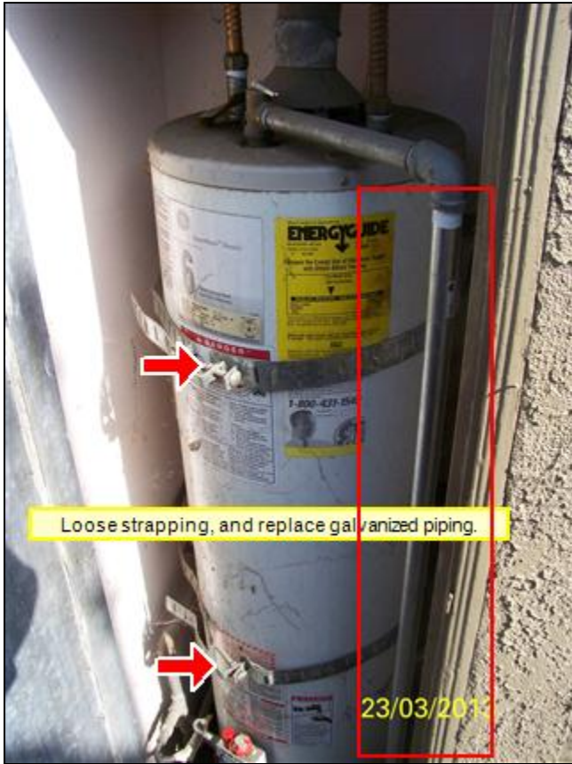
4.2 Picture 1 3707 Water Heater
